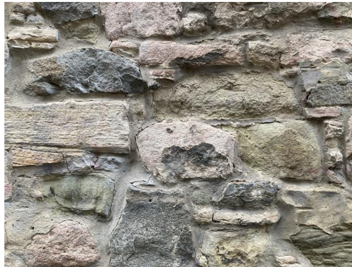
Accelerated stone decay due to cement pointing
