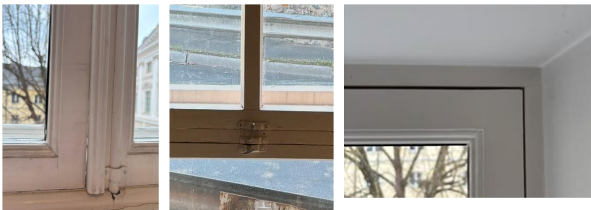
Figure 37 Technical state remarks. See-through cracks (left), missing fastening elements (middle), big gaps between jamb and frame (right)
